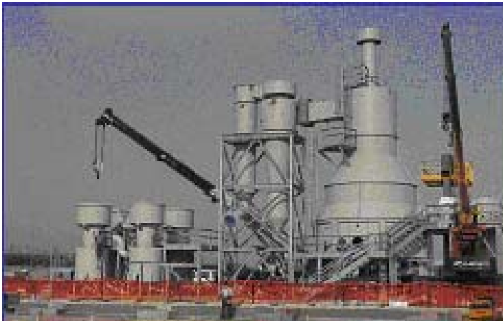
Primenergy Facility in Rossano, Italy
