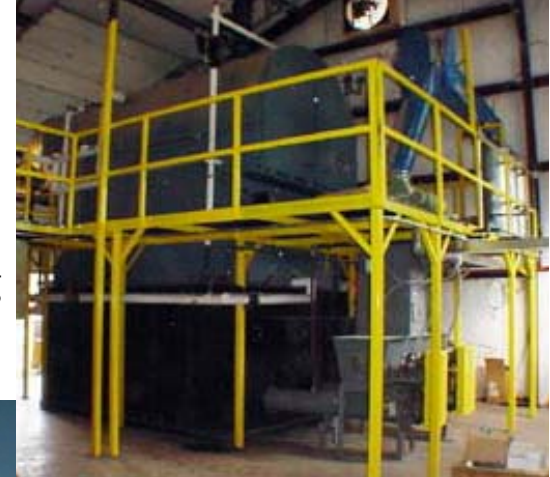
Wood fired boiler generating 12,000 lb/hr process steam
